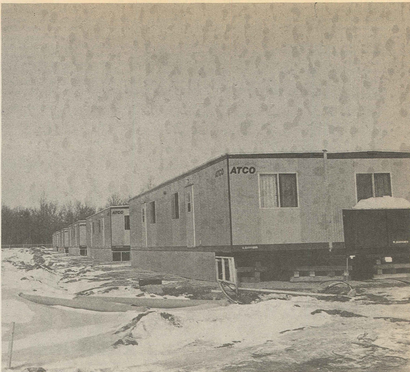
Housing units made by Atco, are erected on the Ain-Ke-Jig site in early March. Atco made the units in a matter of weeks, and
