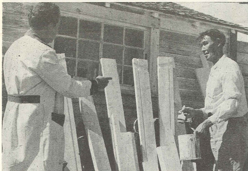
Pierre Marie Niultcho from Dillon paints window frames he has learned to construct.
