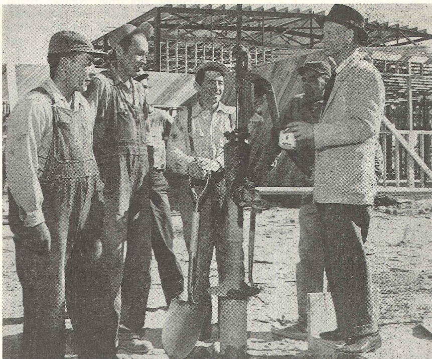
With the exception of a few tradesmen, all workmen helping to build the new Peguis Central school in northern Manitoba are Indians. Here Senator James Gladstone drops in to see how construction is progressing. School, which will have four rooms plus home economics and industrial arts rooms and gymnasium-auditorium, will be completed soon. It is located in the Fisher River Agency. Foundations had to be blasted out of rock and hard pan.
