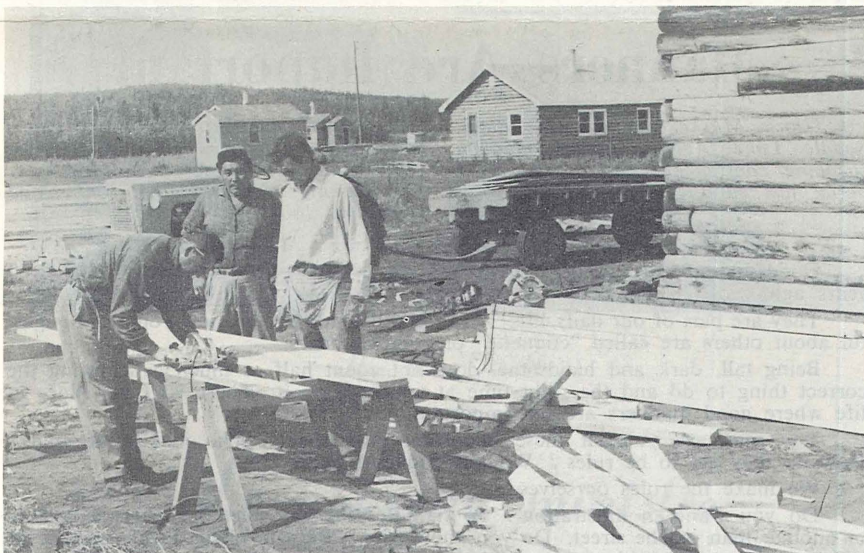
Foreman supervisor, Stan Dutchyshen, (left) is shown with Russel Barker and Antoine Antoine precutting rafters for a new log house at Fort Simpson.
