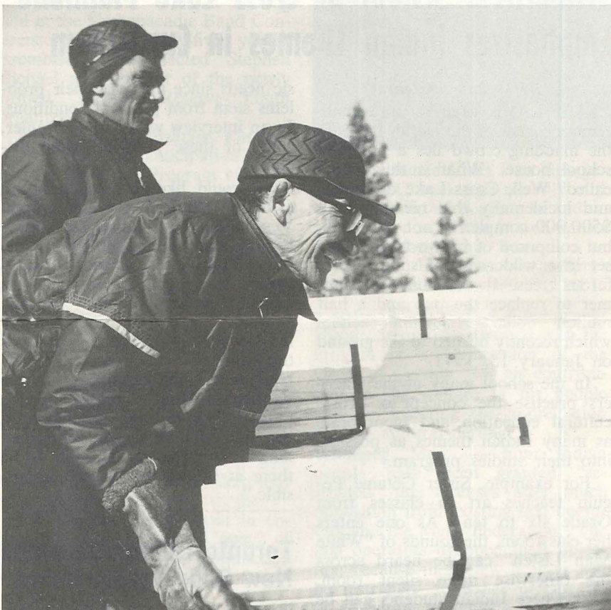
Band members unload first supplies for the two-year project which will provide employment for the Cree community.
