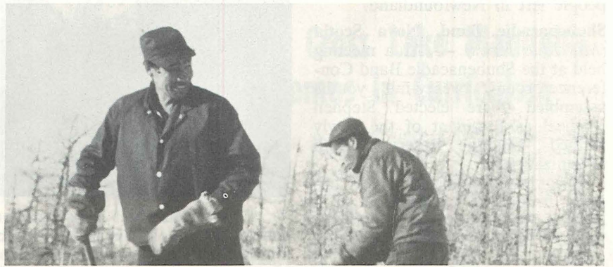
Working in sub-zero cold, band members clear site for school and residence construction which will begin this summer.
