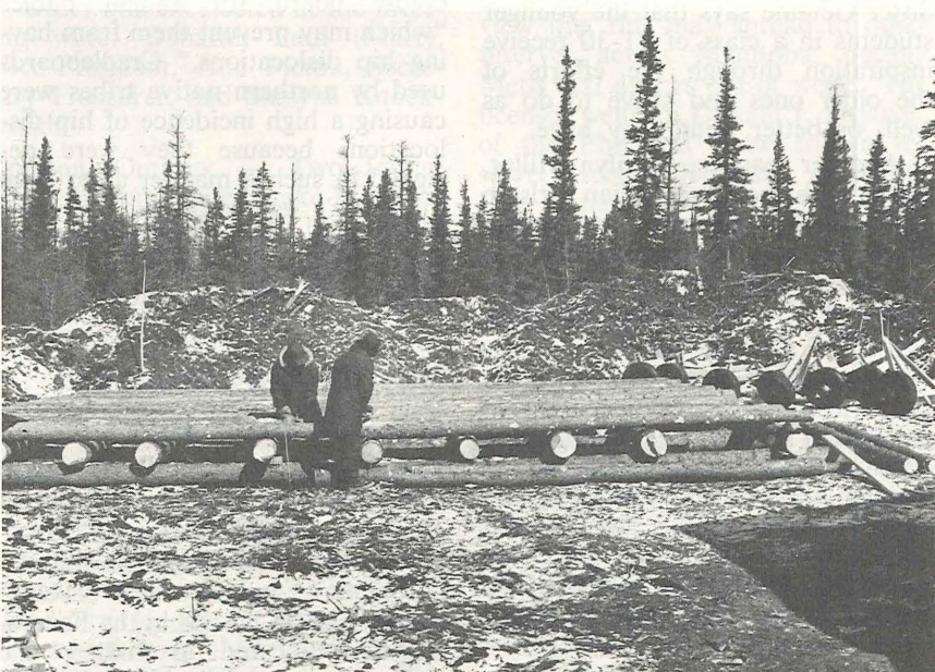
Black spruce trees found in the Albany River area will make suitable supports to prevent a proposed warehouse from sinking into the spongy muskeg.
