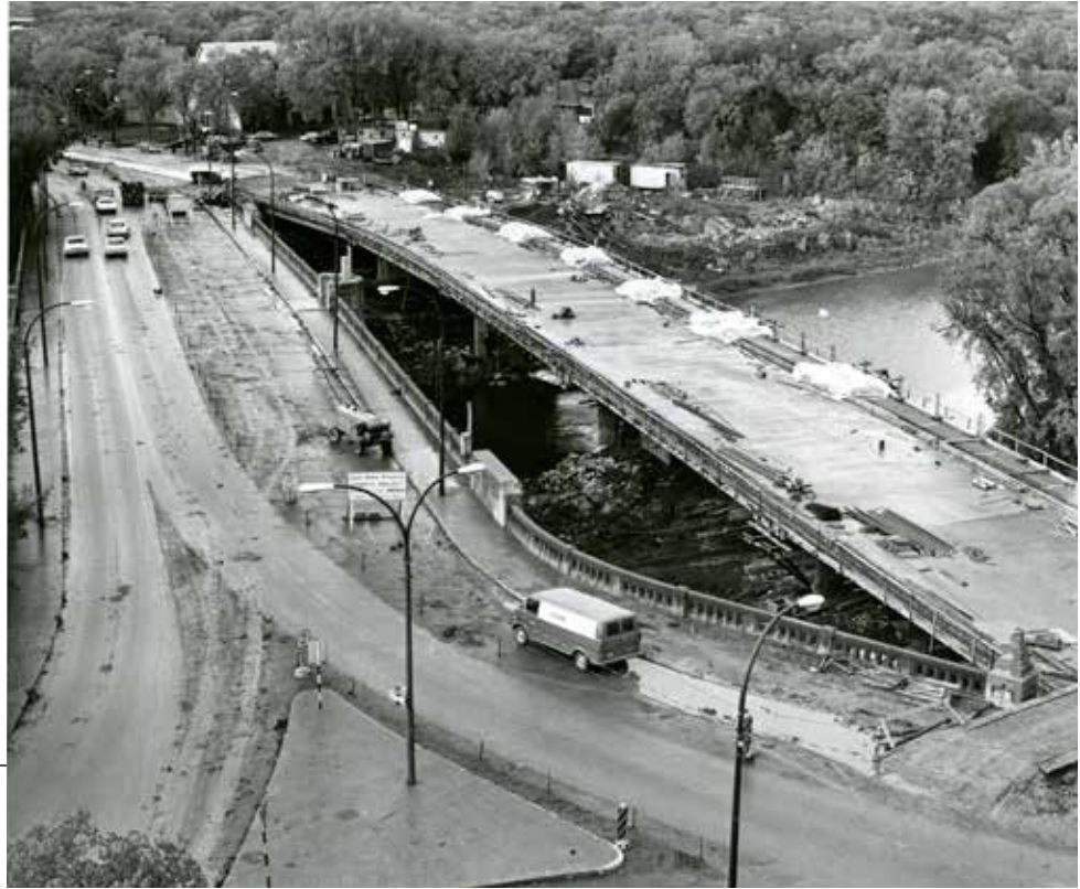
New span of bridge curves into West Broadway (old Maryland Bridge to the left).
