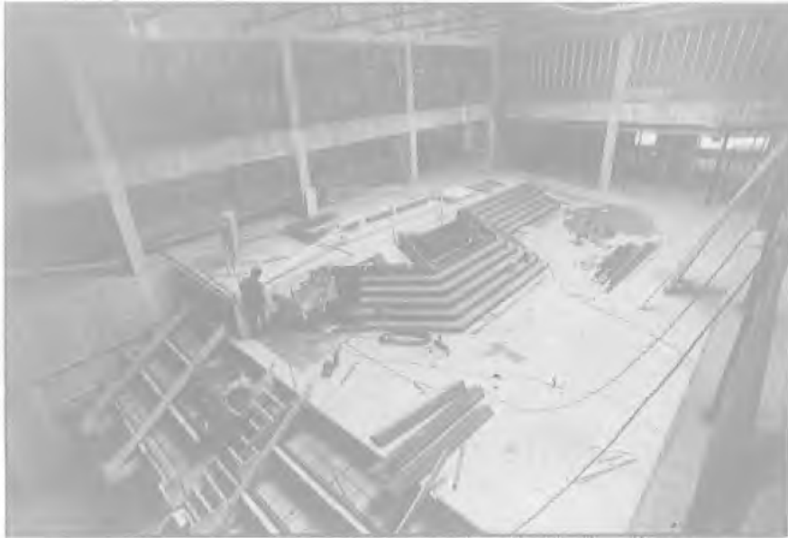
Figure 5. This view, looking down in a north-easterly direction (taken March 5, 1984), shows the steps with viewing-area seats for the handball courts in the foreground, and the upper portion of the gymnasium in the background.
