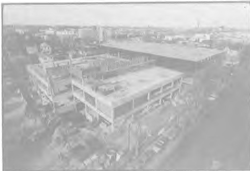
Figure 2. Looking north-westward, this picture taken November 8, 1983 catches the entire complex with external construction partially completed.
