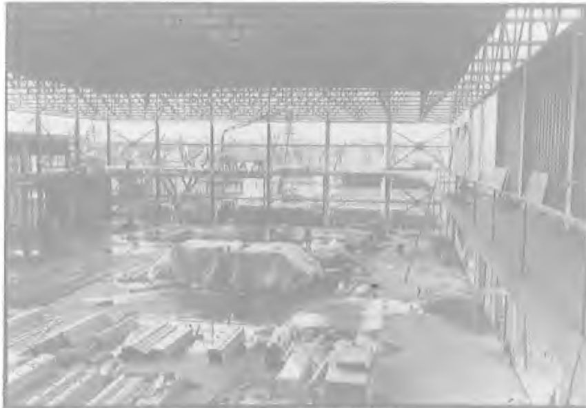
Figure 3. An inside view, looking westward through the gymnasium. The raised jogging track which encircles the auditorium can be clearly seen. The water on the floor created a persistent problem until the roof and walls were completed in early March.
