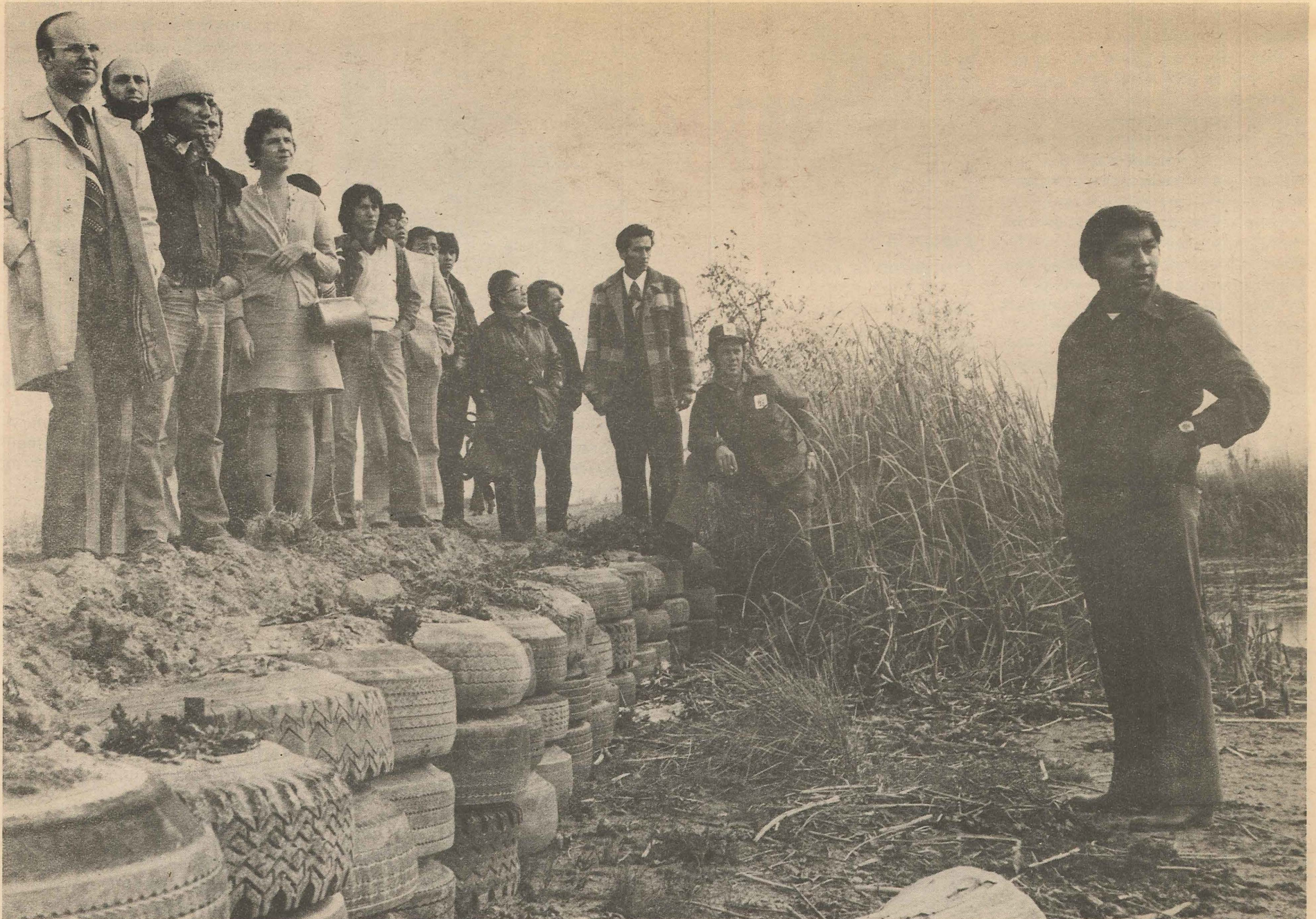
Bill Tooshekenig, right, tells a group of visitors from the press and government about the spring flood that almost wiped out the chance for a crop last year on St. Annes Island. He also showed them an unusual dike construction method using old tires which, to date, has been highly successful. Not only did the Band get in a crop last year, but a bumper crop as well grossing near $500,000.
