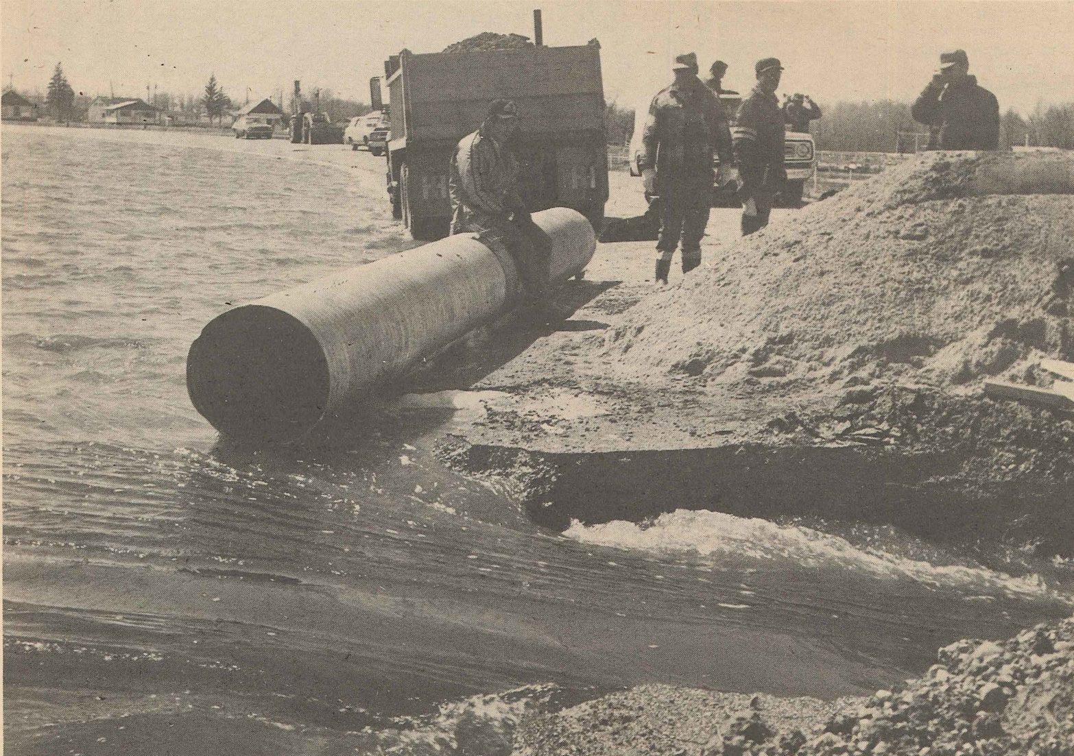
This was the scene on the Peguis reserve on April 29 as flood waters receded and the men were able to return to start the first emergency repairs. One of the first repairs was this break in the highway linking Peguis with
