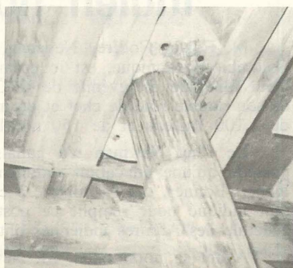
TROUBLE SPOT — The roof beams will likely burn when the stove pipe gets hot.
