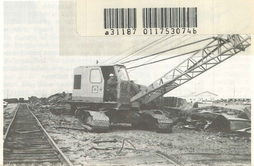
Crane operator Joe Parisien of Fort Qu'Appelle at the controls of the company's 35-ton crane.
